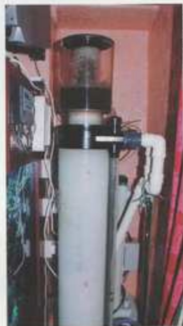
Protein skimmers are at the heart of most big marine systems. This TurboFloater 5000 is being used on Gary's mega reef tank and Mark has two of these on his 7000 Lt tank.
